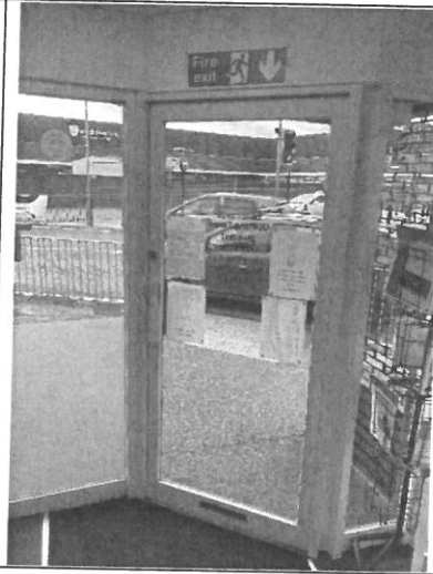
20 – Entrance to the public is controlled by staff using a key. Alternate fire exits available with push bar to open at rear
