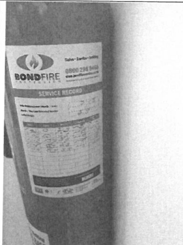
12- Fire extinguisher tested annually
