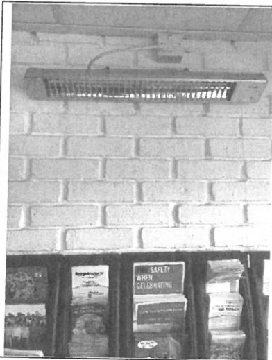
19- Radiant bar light in main entrance requires strict controls as evident here keeping clear space on the wall
