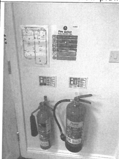
6- Unit 13- Fire point
